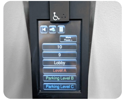
Destination elevator touchscreen
